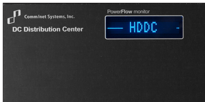
Figure 2. HDDC Supervisory Control Panel
