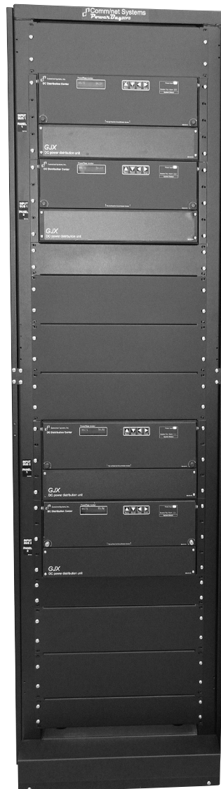
Figure 2. Dual Bus BDFB Cabinet
